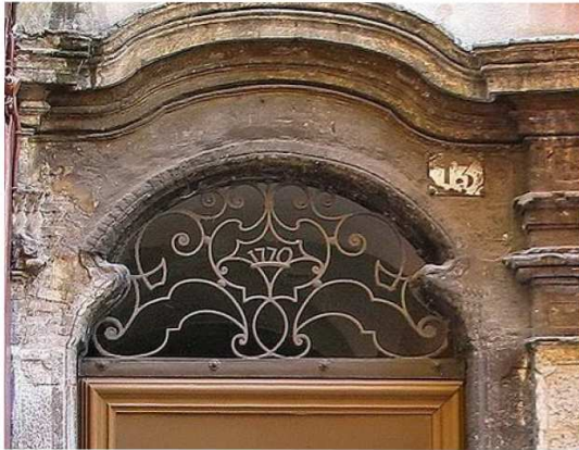
Ventilation Vieux Nice
